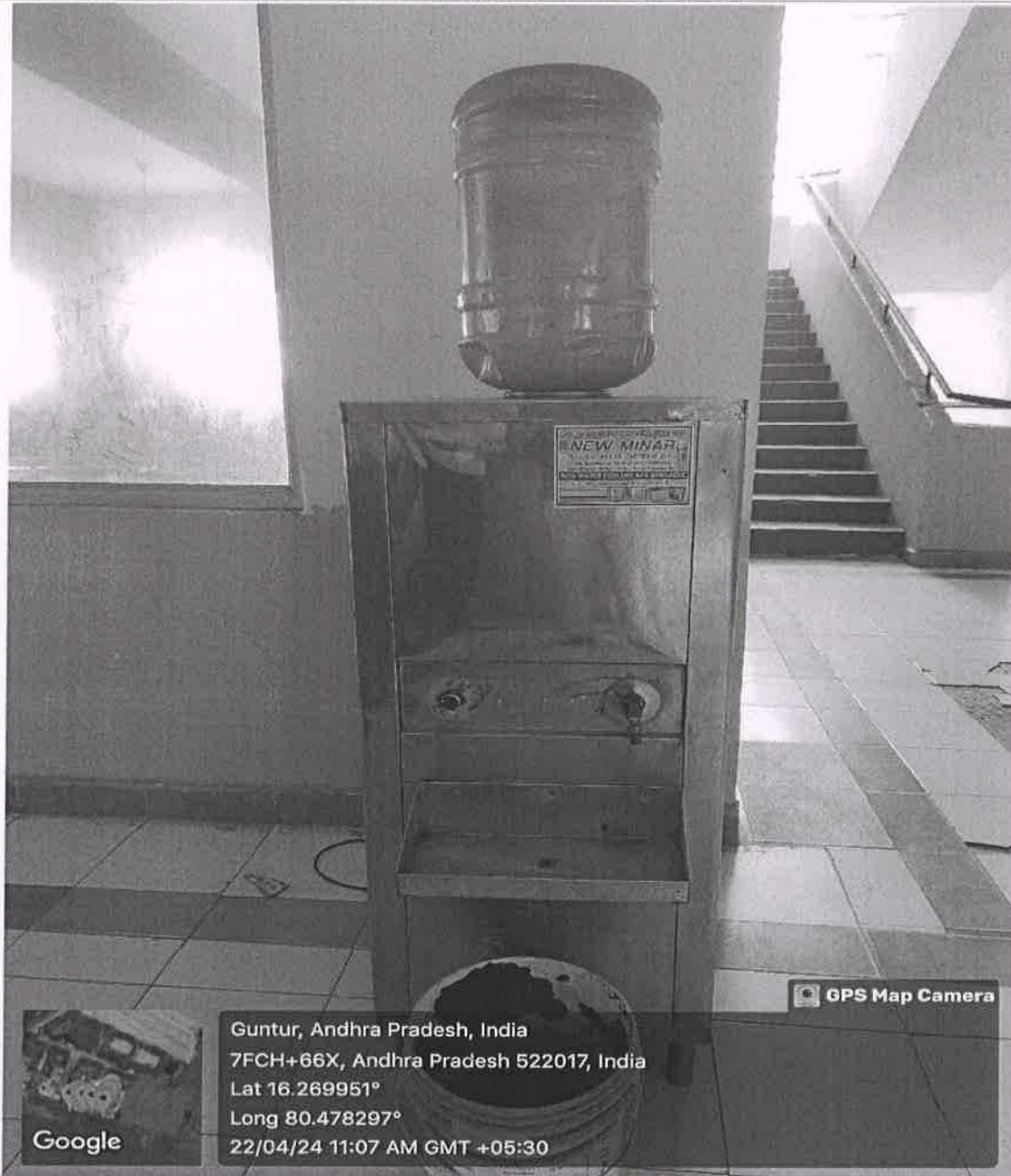
Drinking water facility
